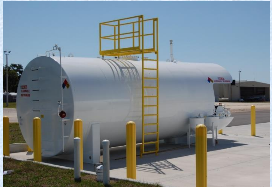
Fuel Storage Tank
